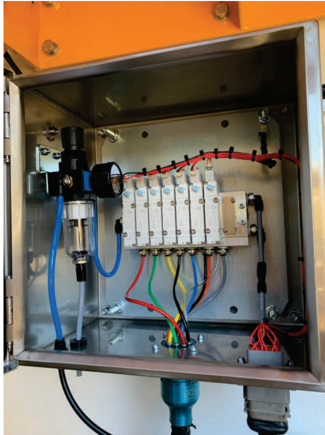
Figure 15. Air solenoid control box, key in cab
