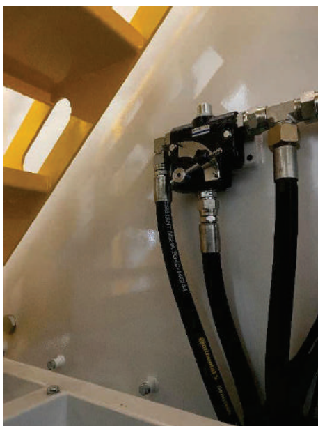
Figure 9. Flow control valve under the steps
