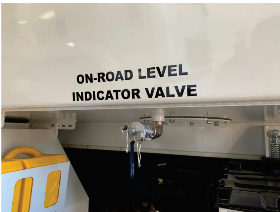
Figure 18. On-road Level Indicator Valve
