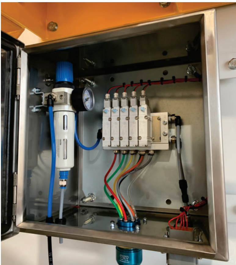
Figure 17. Air solenoid control box, key in cab
