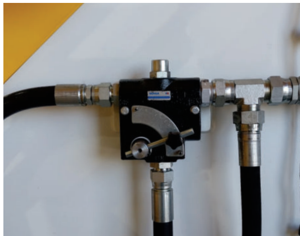
Figure 9. Flow control valve under the steps Preset for ideal cannon pressure; please do not adjust.
