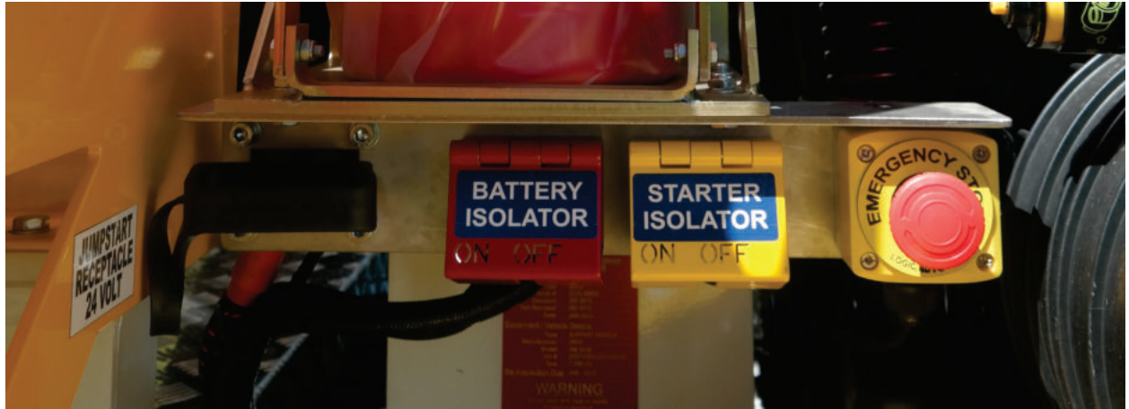
Figure 14. Jumpstart Receptacle, Isolators and Emergency Stop
